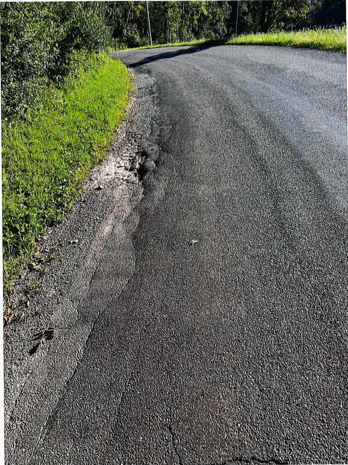
Photo 9 – Phineyville Road (T-875) – Typical Lack of Adequate Sight Distance/Shoulder Deterioration
